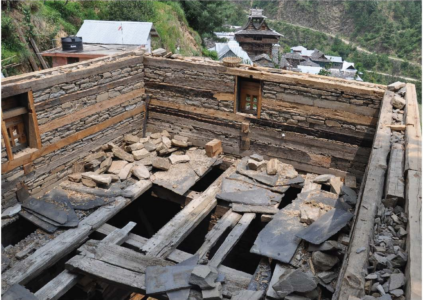
101. Kath-khuni wall construction. Dry masonry wood-and-stone wall of a temple under construction in Devidhar. This infill is filled with stone rubble.
